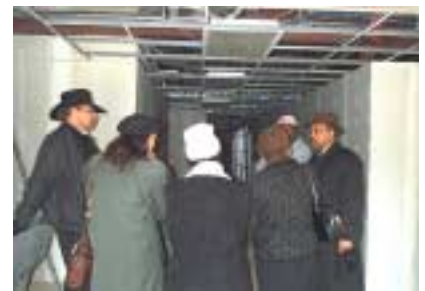
UPO's Wayne Thompson, wearing hat at right, discusses building progress during one of many, many staff visits to headquarters construction site.
